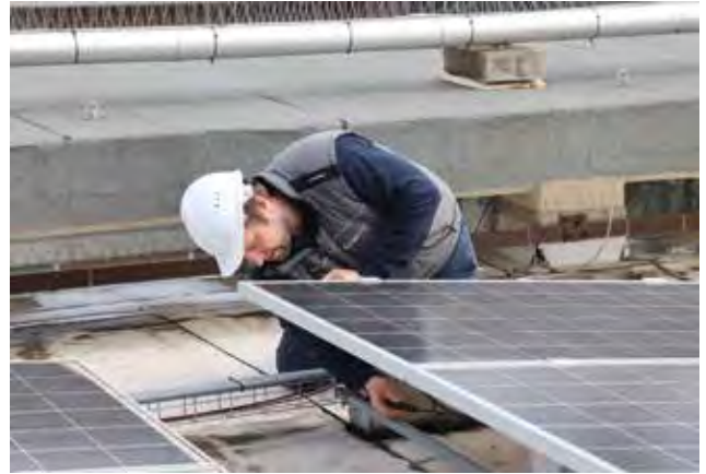
Maintenance services, Borgo Roma Hospital – Verona (Italy)
