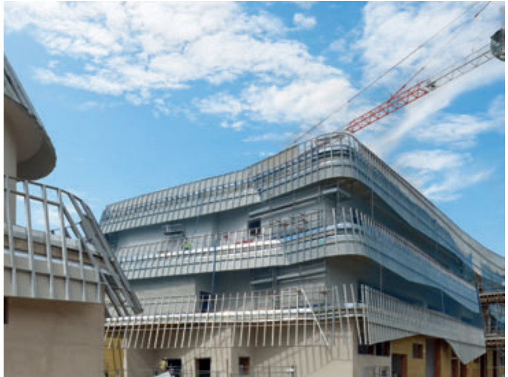
Borgo Panigale tram depot — Bologna (Italy)
